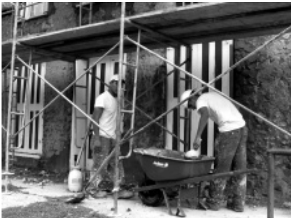
Workers from Simpson Plastering Co. remove and replace the exterior stucco on the Trade Center. The restoration should help preserve the building for another 164 years.
